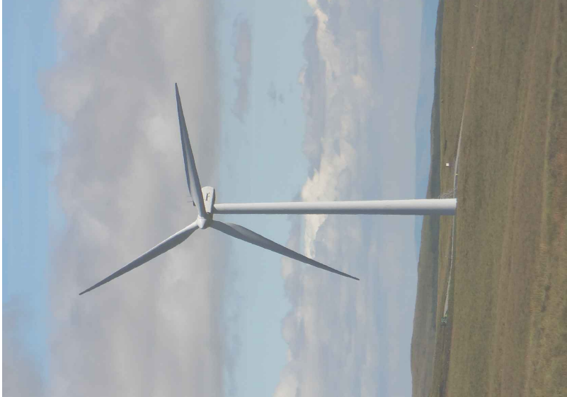
PHOTOGRAPH OF TYPICAL TURBINE
